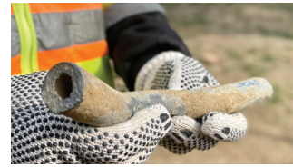
Lead water service line
