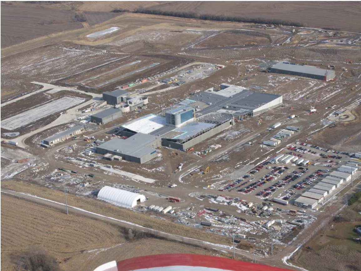
Water Treatment Plant (Taken December 3, 2007) Aerial View Looking Northeast (Intersection of 216 th and Q Streets in lower left corner)
